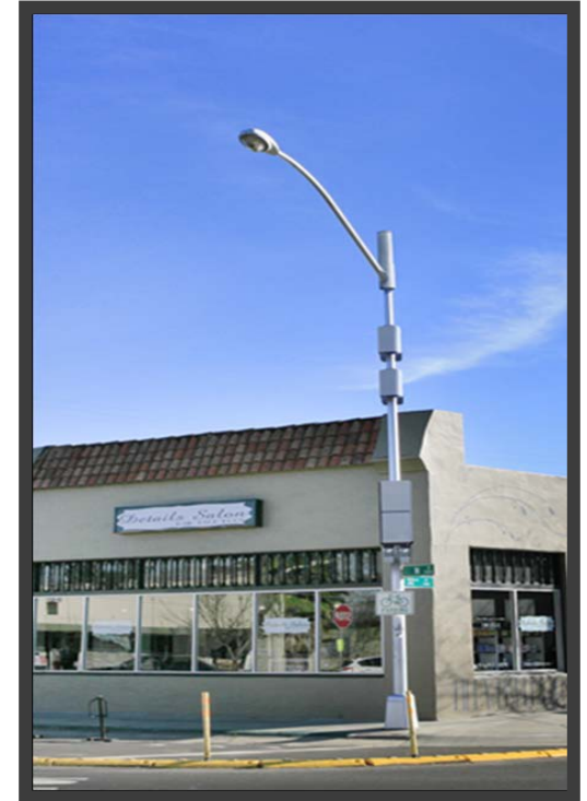
Pole-mounted battery backup
