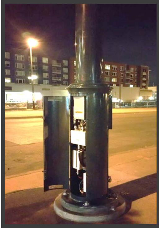
Equipment inside of pole base
